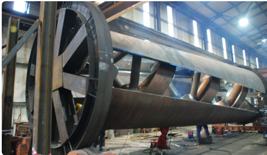
Steel fabrication of the towers in Bolton. Image courtesy of George Oates, Expedition Engineering
